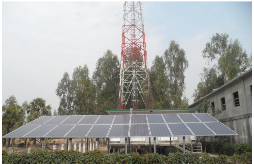
Solar Power for BTS Station installed by Allied Solar Energy Ltd. at Brindaban, Bogra
